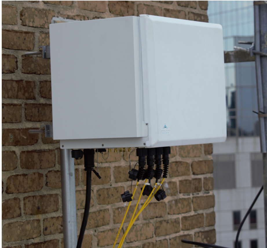
Figure 5.9 : Single 160-radio CBRS weatherproof ArgosV3 base station mounted outdoors. Four single-mode fiber pairs provide up to 40 Gbps connectivity.
